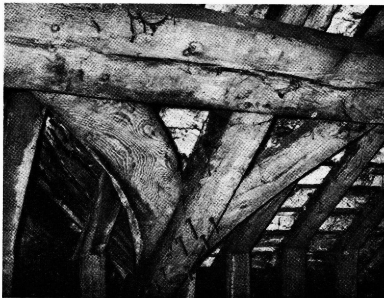
FIG. 14. The subsidiary principal rafter. DETAILS OF WEST SIDE OF SOLAR ROOF, CHORLEY HALL.
